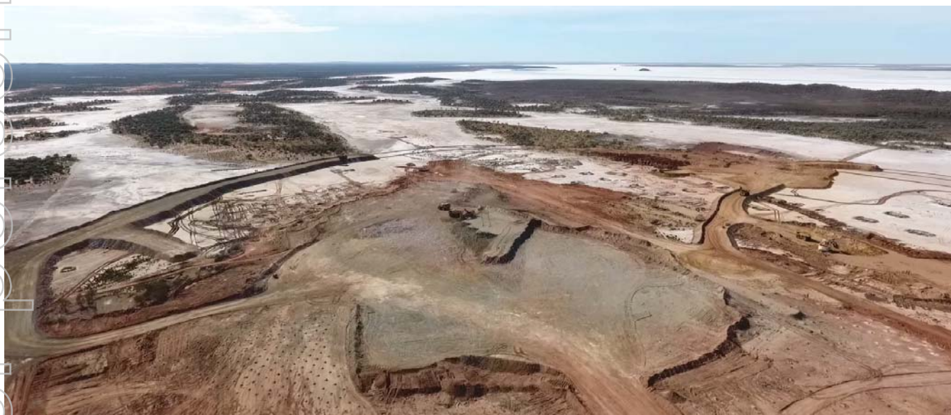
Figure 6: Open pit mining at Jupiter has commenced with mining of the top 15m off Heffernans Hill.
