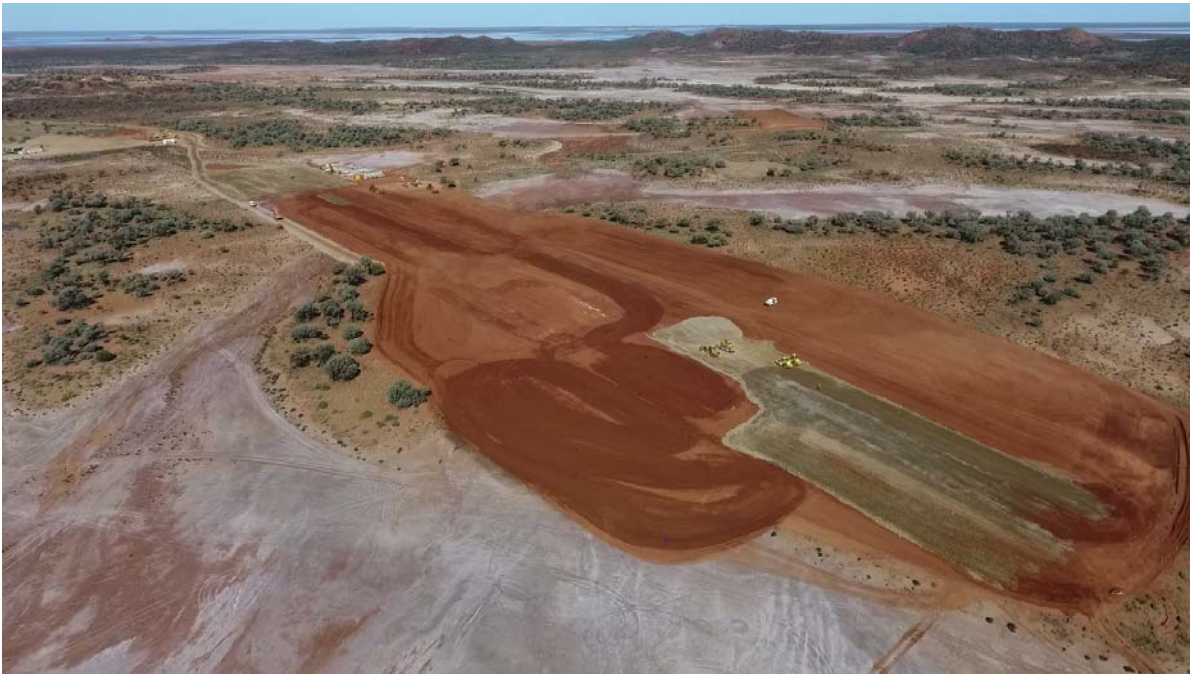
Figure 2: Photograph showing the cleared area and construction of the pad for the 2.5Mtpa treatment plant. The photograph was taken on the 24 th May 2017.
