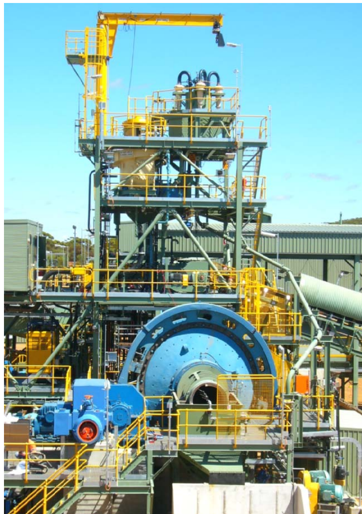
Figure 3. Ball mill, cyclone and control room
