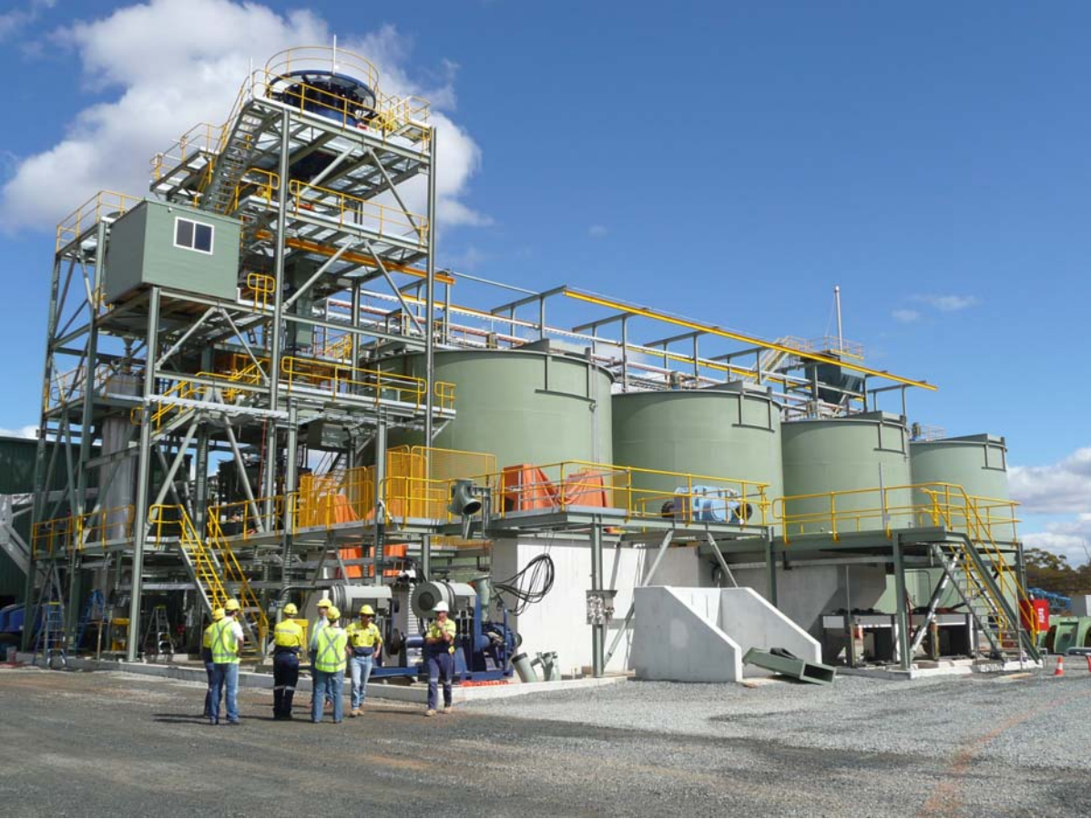
Figure 3: Leach and elution circuits at the Higginsville treatment plant. Ball mill is to be placed on the concrete footings in the foreground.
